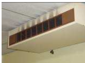
Figure 11 : Installation de chauffage mal entretenue (Corenc).
